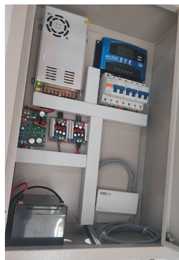
(c) Battery storage system and POE switch
